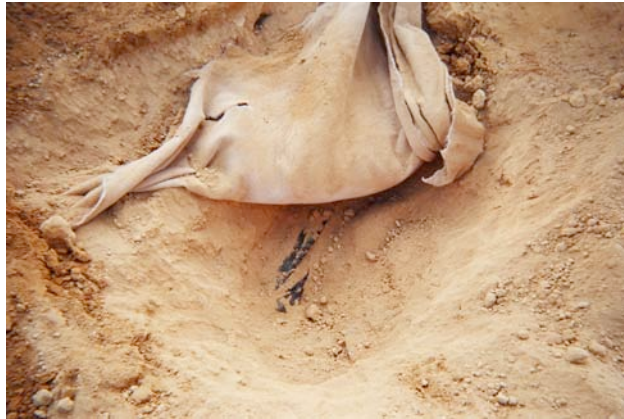
Figure 5. A one meter tear discovered using the dipole method, caused by heavy equipment during covering material placement.
